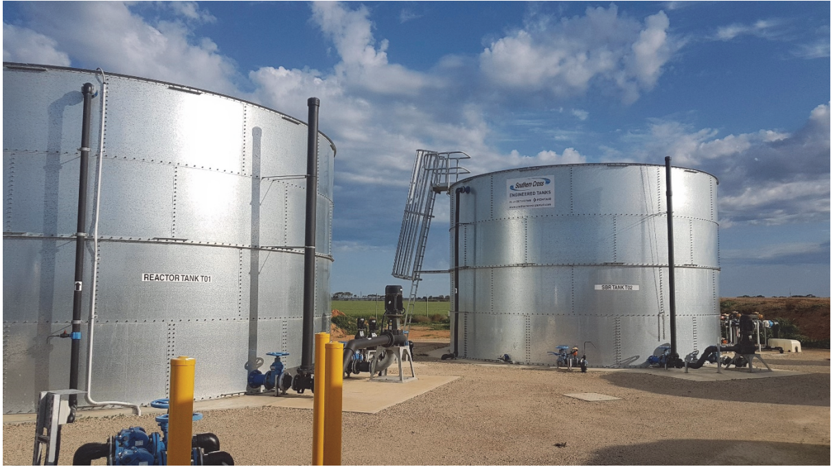
Mallala Council's wastewater treatment plant's treatment tanks. The CWMS scheme cost $6.9 million.
