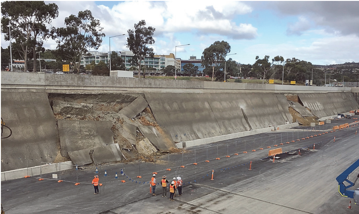
Figure 4.2: Retevment wall slumps on eastern section of the lowered motorway
