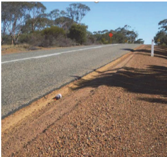
Damaged edge causing a drop off (safety issue)
