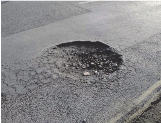
A pothole with cracking
