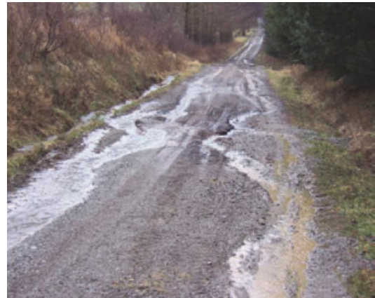
Deformation (washout) due to flooding
